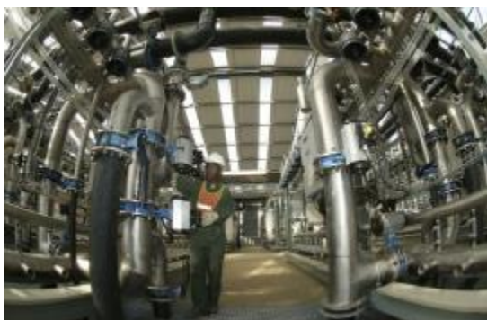
Anglo American eMalahleni Water Reclamation Plant
