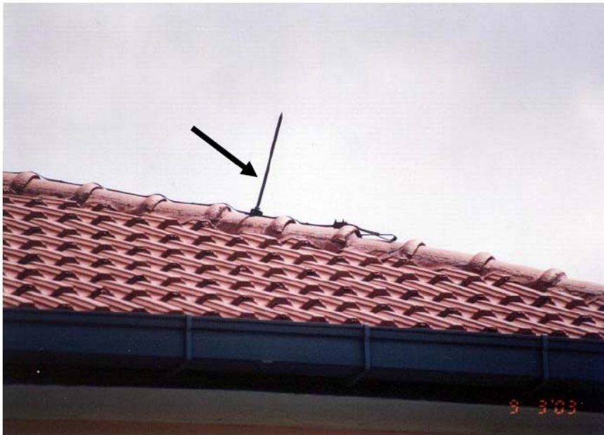
The typical conventional air terminal or Franklin rod (arrowed) which had been installed on the roof of a building. It can either have a sharp or blunt tip (preferred).
