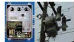
Switched Cap Banks
