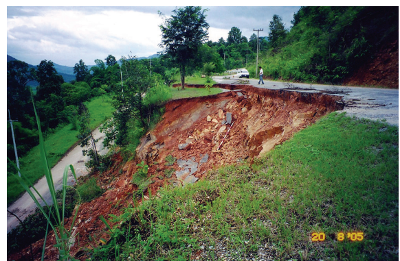
Figure 2: Failure of the access road.
